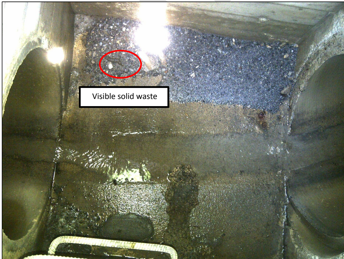
Figure 4: 350 Chelsea Rd – Solid waste visible in manhole
