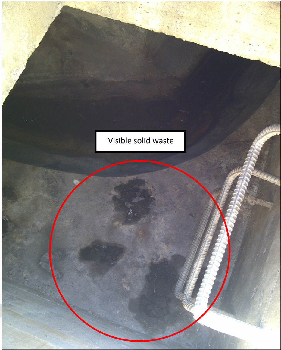
Figure 5: 373 Chelsea Rd – Solid waste visible in manhole
