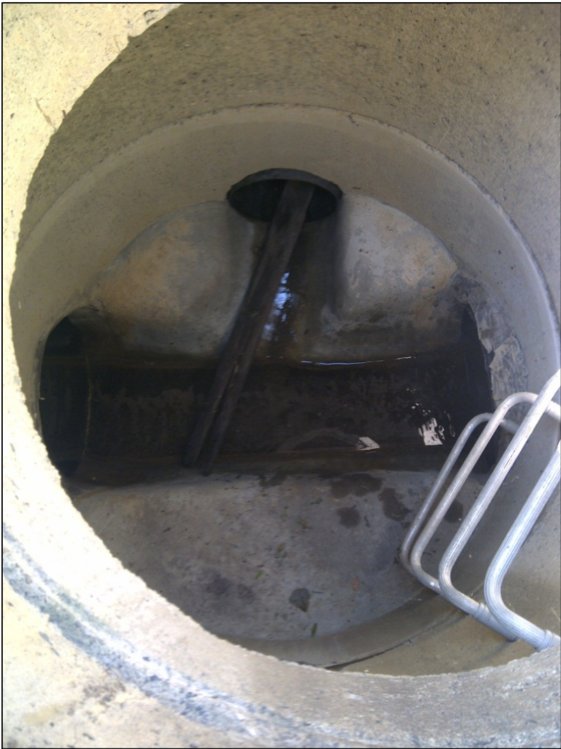
Figure 9: 15-102MH3-1 – Lydia Crt. and Katherine Street – Wood debris
