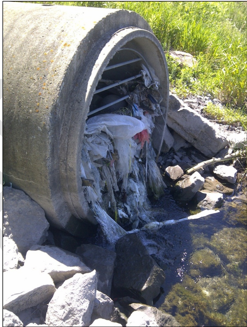
Figure 10: OF 249 – Garbage and Debris Clogging Outfall
