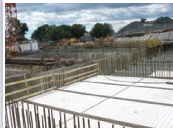
Early stages of BAF cells showing inlets for some of the 77,000 nozzles.
