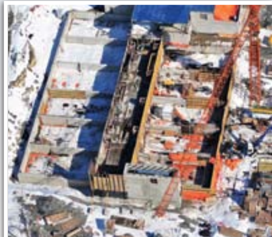
Eleven cell BAF has a footprint of 1500 sq metres for the cells and an overall area of 3000 sq m.
